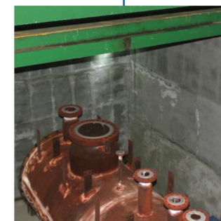
Underground RT Room 6M x 6M x 12M
